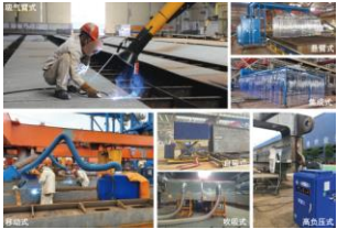
Welding Smoke Control
